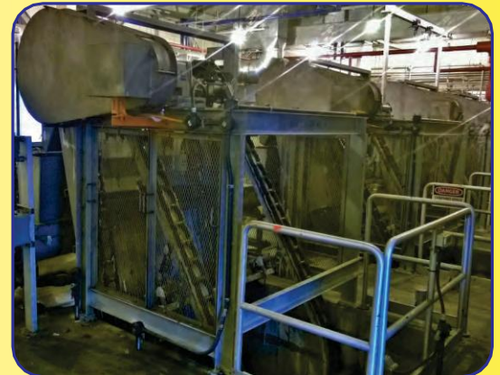
Catenary Bar Screen
